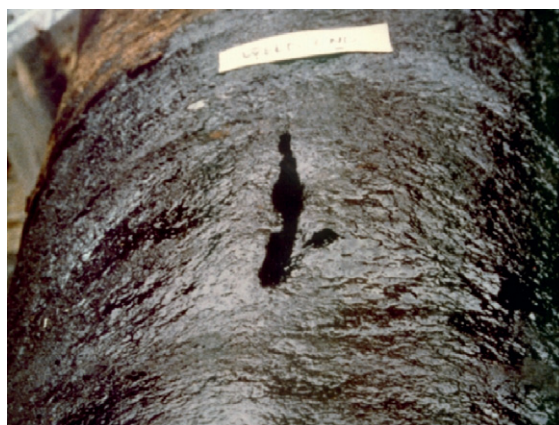
Figure 2 Burst failure of carbon steel oil pipeline (due to lack of cathodic protection).
