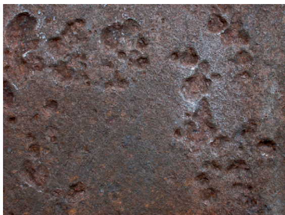
Figure 4 Typical morphology of SRB-mediated MIC of carbon steel, an example from sheet steel piling.
