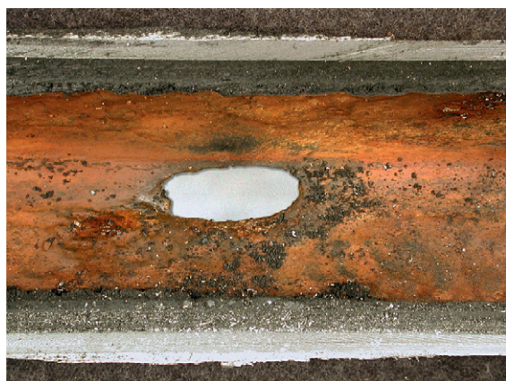
Figure 8 SRB-mediated internal MIC of an oilfield water gathering line.
