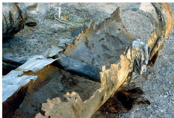
Figure 12 Corrosion of a mortar-lined ductile iron wastewater pipe because of activity of Thiobacillus .
