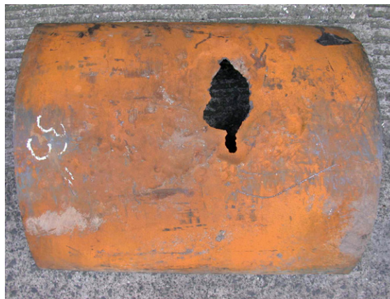
Figure 1 Corrosion of cast iron pipe (due to external stray current).
